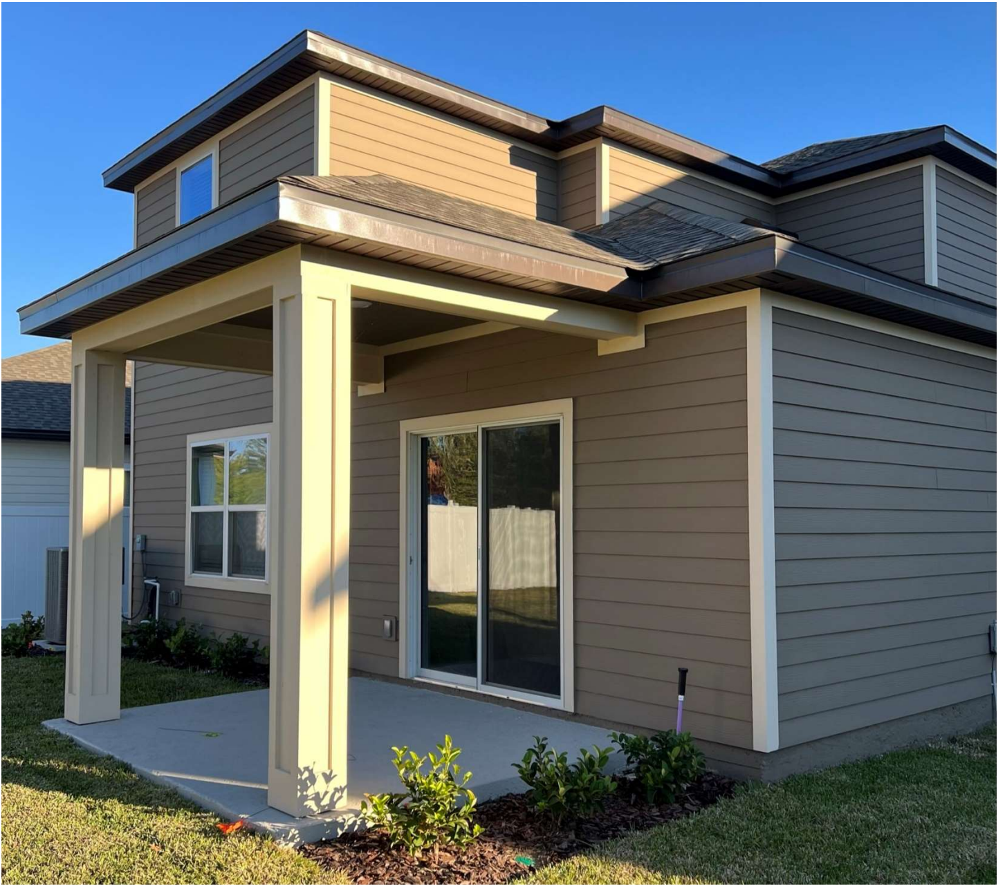
Rear patio roof line without rain gutter.
