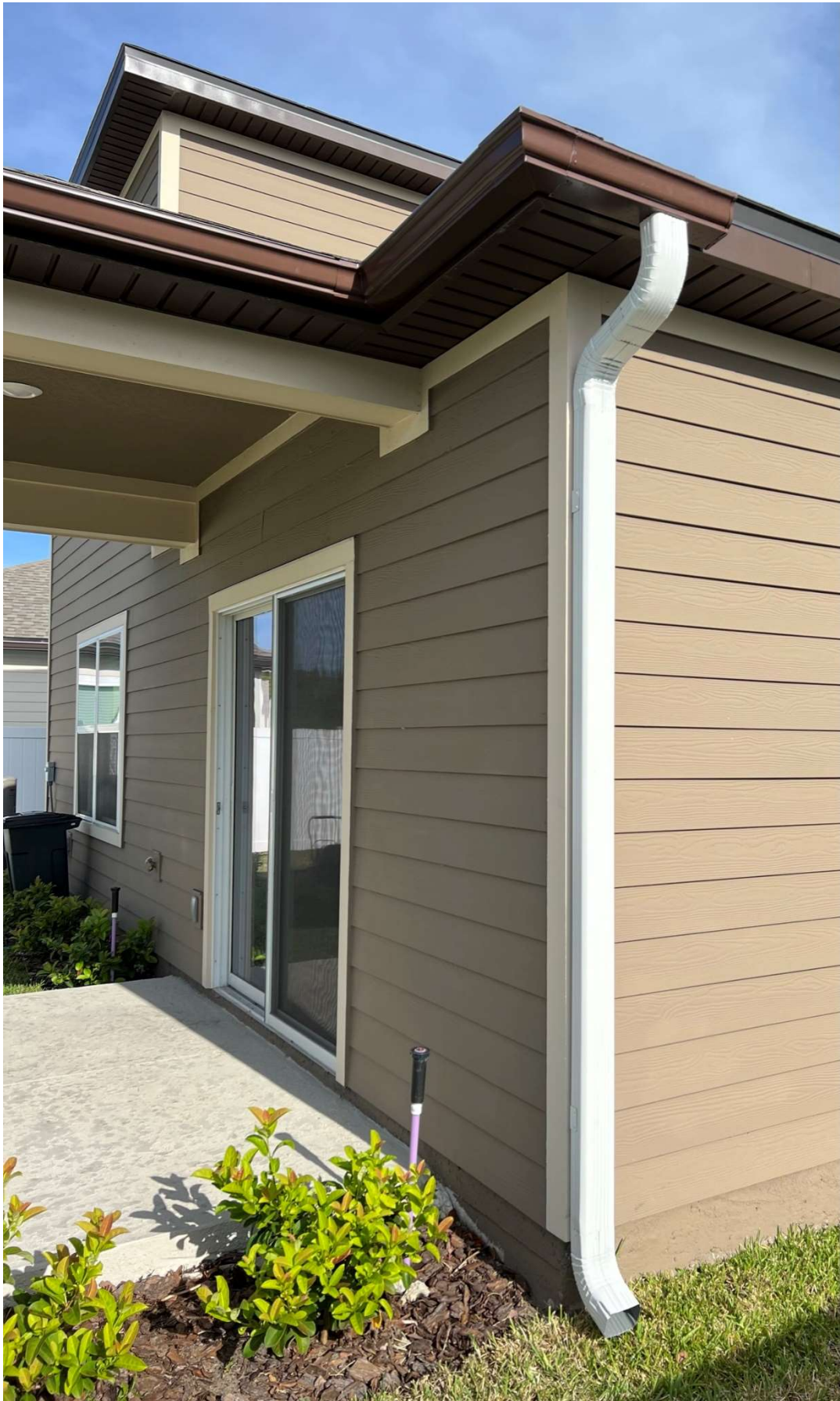
Rain gutter down spout.
