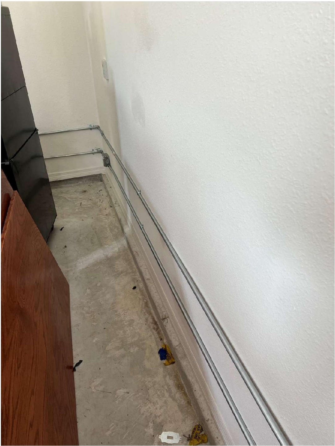
A 120VAC 4 plex outlet shown in the corner.
