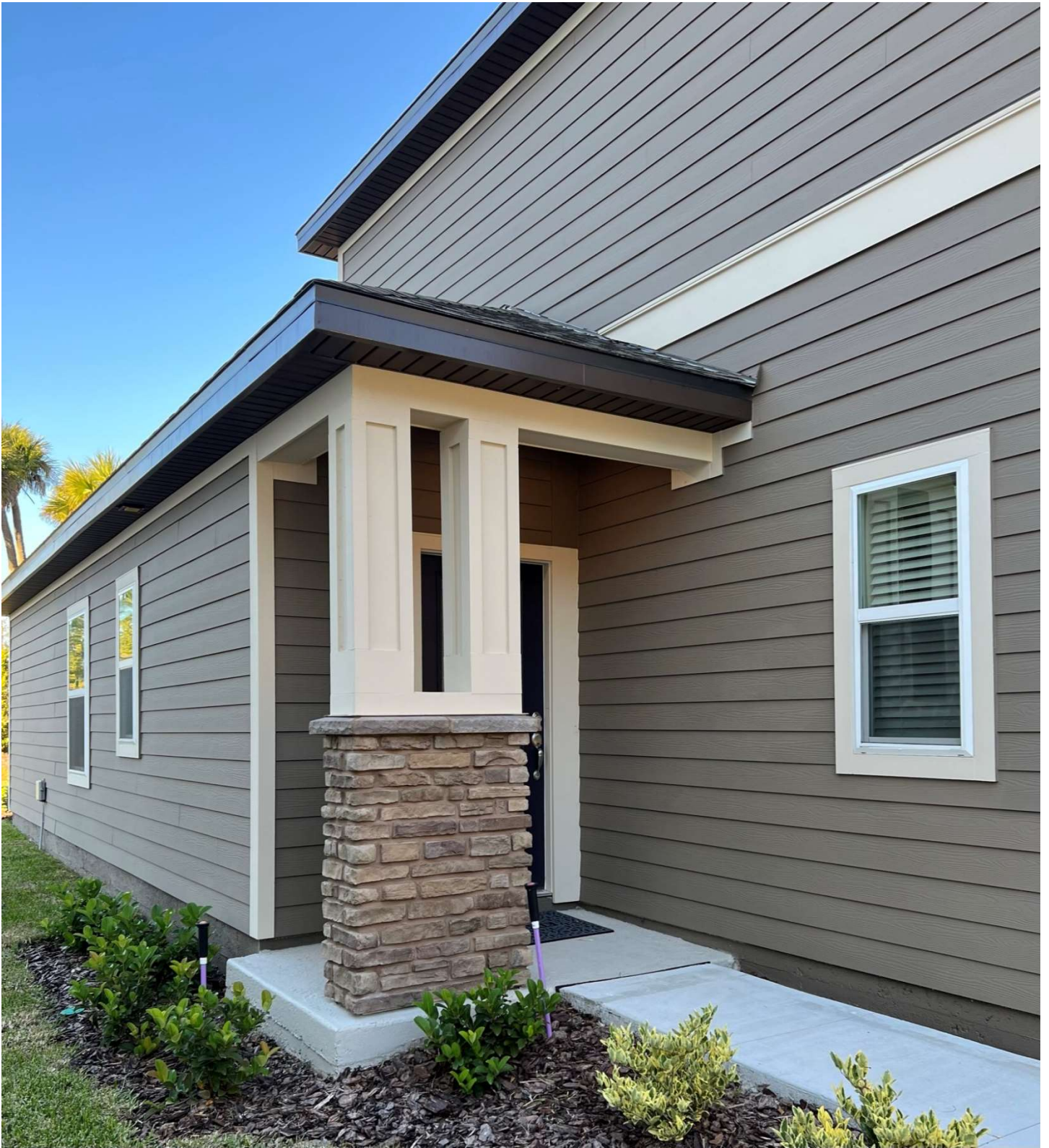
Front porch before rain gutter.
